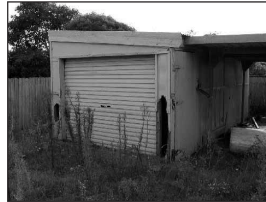
These old sheds and garages can be found in backyards Australia wide. Asbestos was also commonly used to build bungalows.
