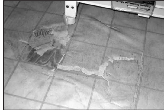
Vinyl itself does not usually contain asbestos. It is in the white backing material that can be seen here where the vinyl has worn through.
