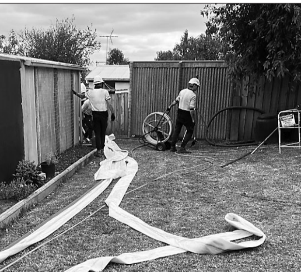
Then the resin saturated pipe was inflated and installed into the pipe.
