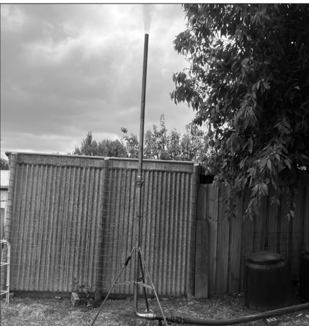
It was then cured with steam. A small chimney removed the smoke.
