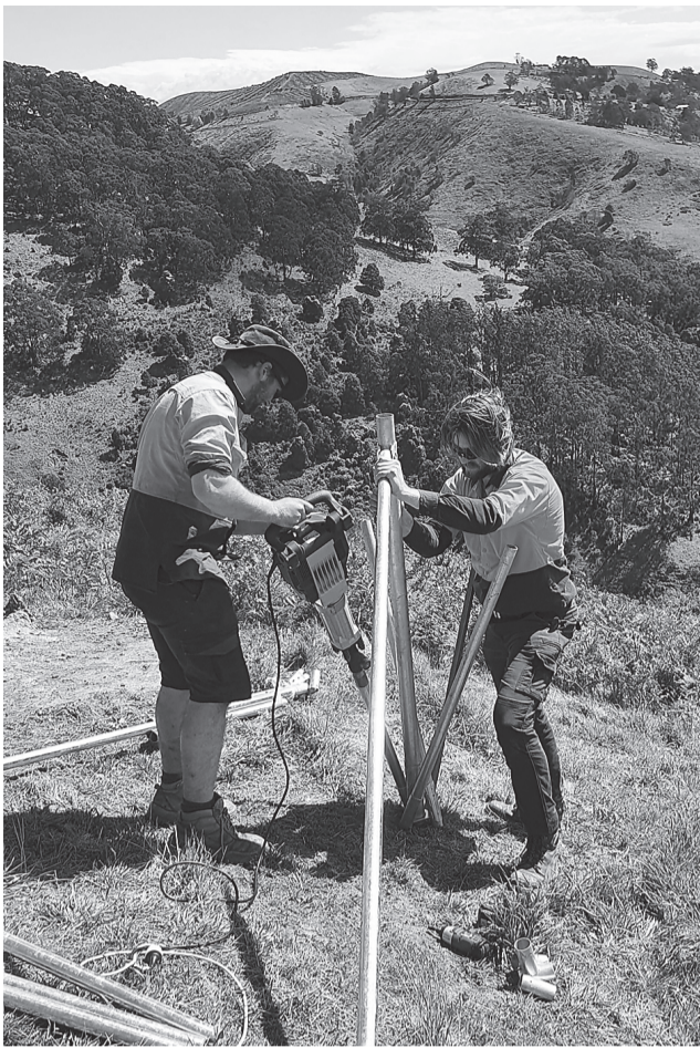
Our last stand against the deer. Contractors installing our browser fence at Billys Creek
