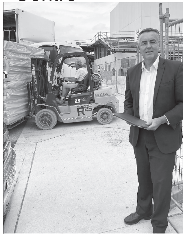
Federal Member for Gippsland Darren Chester said works to fit out the interior shell of the Gippsland Performing Arts Centre were underway. Please note: Mr Chester is pictured prior to the stay at home and masks requirements being implemented.
