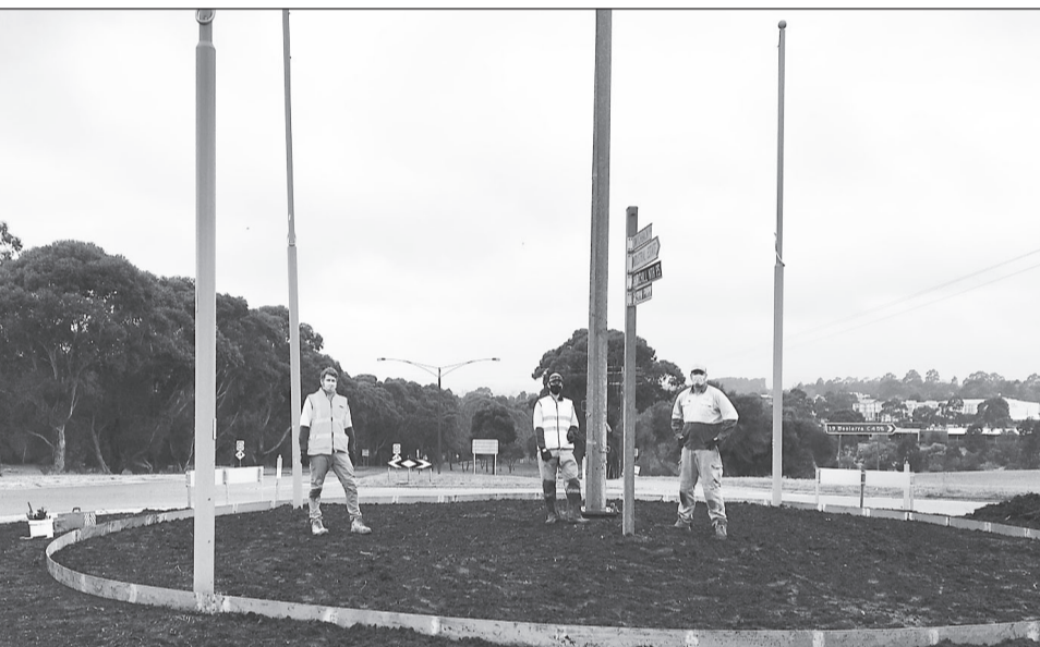
Work is being carried out on the grounds surrounding the roundabout. By the time the paper is published we should see what is to be the outcome.
