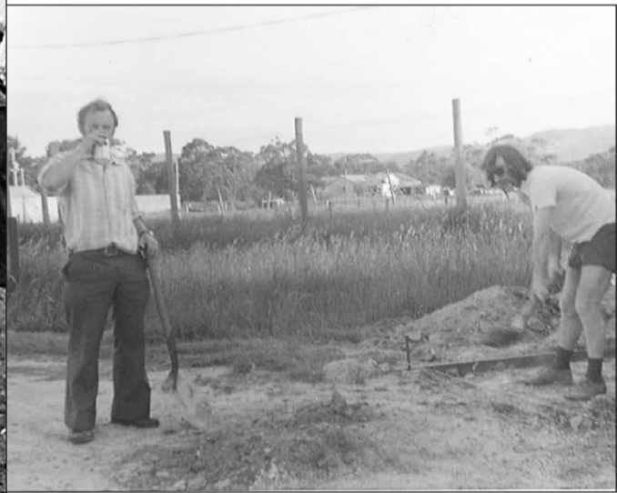
Frank Johns and Bob Rodden preparing the concrete reinforcement in front of the J. Silcock Pavilion in late 1972.
