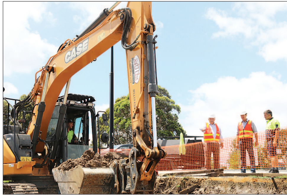
Latrobe City Mayor Councillor Darrell White, inspects the works at Latrobe Synthetic Sports Field Pavilion, Churchill with Latrobe City building projects officer Geoff Derham and contractor Rick Doultree from Rick Doultree Builders.
