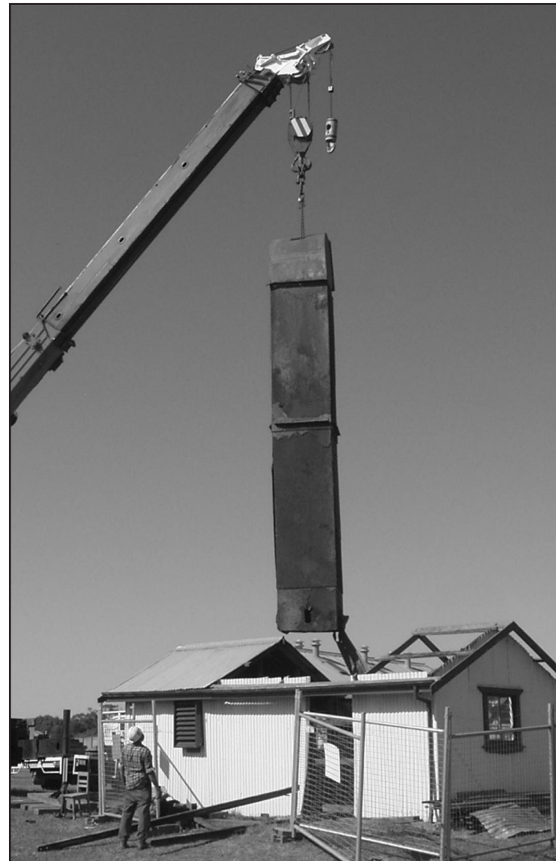
Wonthaggi Mine: the 7 metres long ventilation shaft liner emerges from the dark
