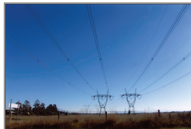
Power Poles Tom Mikulic
